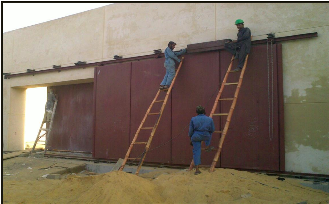
Figure 8: Automatic Heavy Steel Gates
